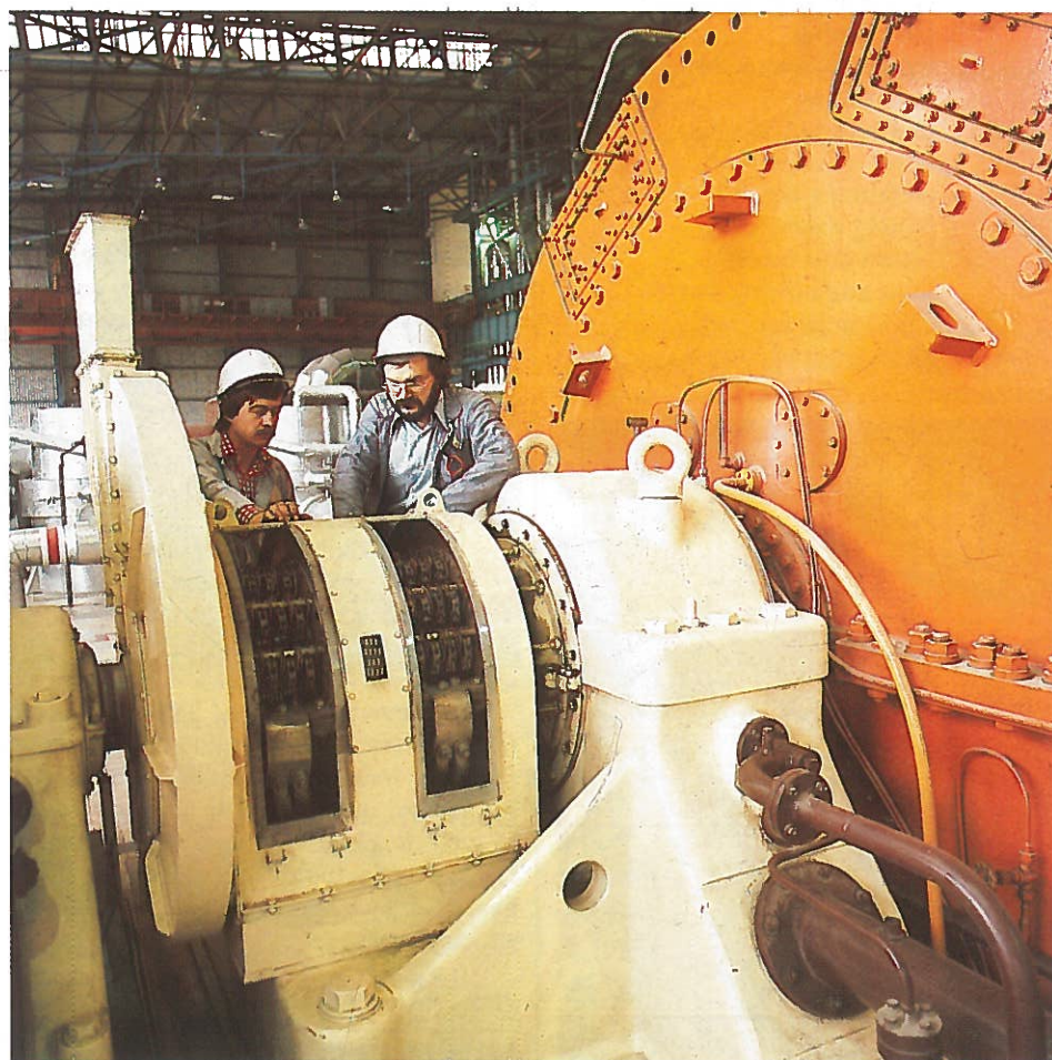
The power station Pruněřov II - a part of one turbine unit in the machine-hall
